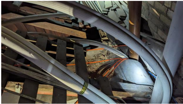
Figure 3. Original cut rafters for service penetrations
